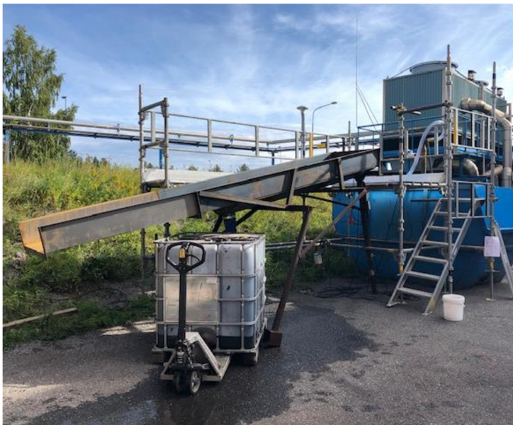
Figure 12. Installation of a sieving table and stirring of blast furnace sludge in a container.
