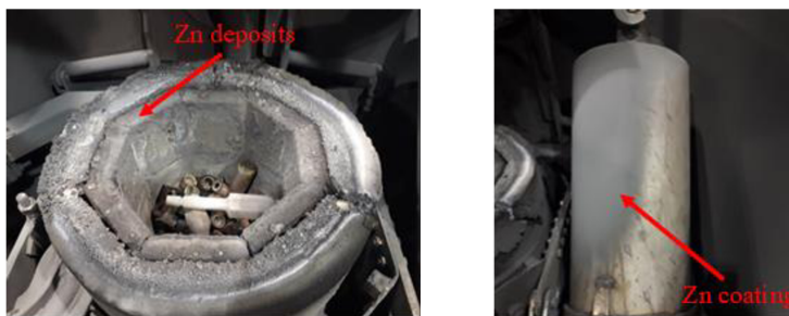
Figure 3 Zn deposits and coatings due to escaped vapour
